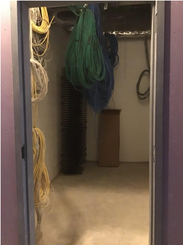
IT Room with Bundled Network Cables
